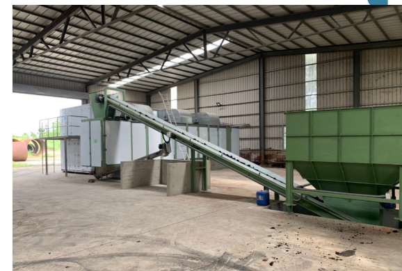
Sludge Reduction Equipmen
