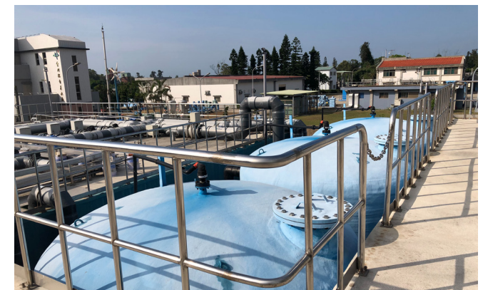
Kinmen (4000 CMD) Seawater Desalination Plant
