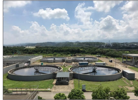
Zhunan Toufen Water Resource Recovery Center (Secondary Sedimentation Tank)
