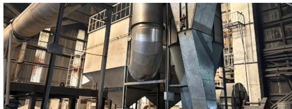
Exhaust collection piping
