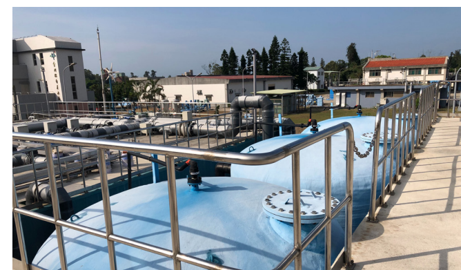
Greater Kinmen Seawater Desalination Plant (4,000 CMD)
