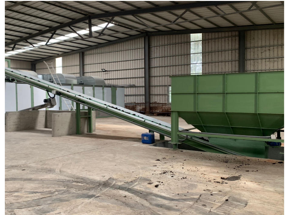
Sludge Reduction Equipmen
