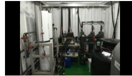
Inside of Container 貨櫃內設備
